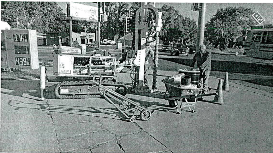
PROJECT: Illinois Ayers Oil Company-Springfield PHOTOGRAPH #8 DATE: 8/31/23 VIEW: North DESCRIPTION: Drilling Monitoring Well PMW-24.
