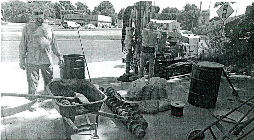
PROJECT: Illinois Ayers Oil Company-Springfield PHOTOGRAPH #12 DATE: 8/31/23 VIEW: East DESCRIPTION: Drilling Monitoring Well PMW-26.
