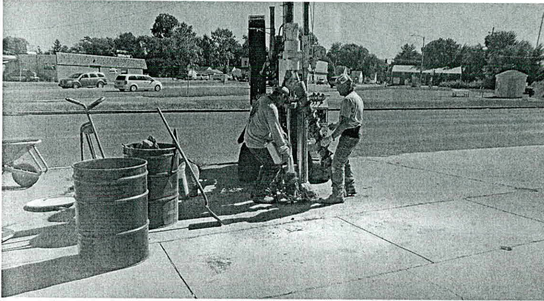
PROJECT: Illinois Ayers Oil Company-Springfield PHOTOGRAPH #11 DATE: 8/31/23 VIEW: East DESCRIPTION: Installing Monitoring Well PMW-25.
