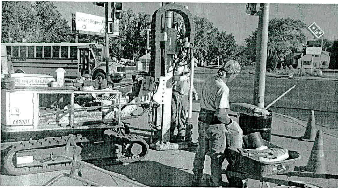
PROJECT: Illinois Ayers Oil Company-Springfield PHOTOGRAPH #9 DATE: 8/31/23 VIEW: North DESCRIPTION: Installing Monitoring Well PMW-24.
